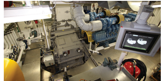
Looking down to port and starboard views of the engine room.
