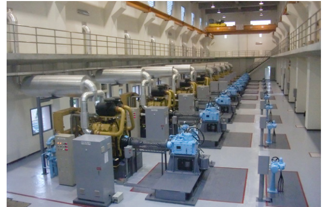
The Jingmei pumping station uses a lineup of CAT engines with Logan Bell-Housing PTO clutches to power their pumps
