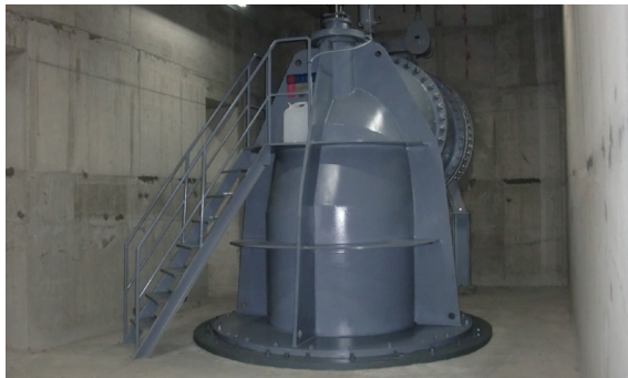
Large pumps are required in order to reach a total output of 95,000 gallons / 360 cubic meters per min
