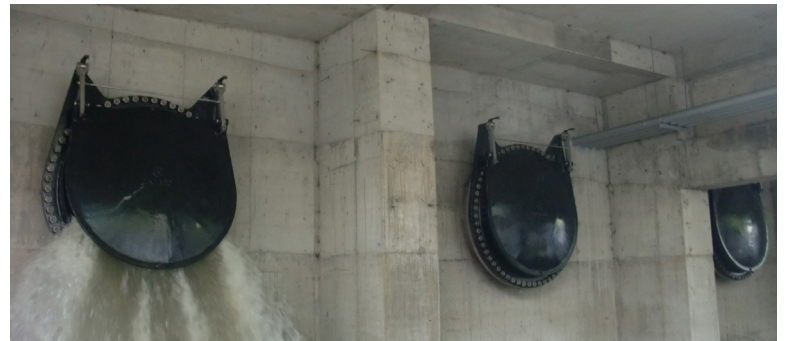
Pumping stations are critical during the rainy summer and autumn months in Taipei to move huge amounts of water
