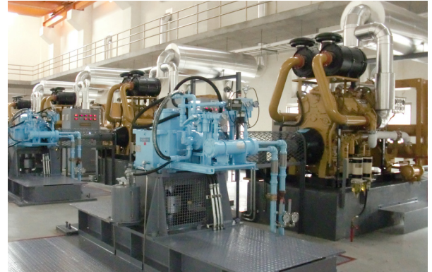
The Logan LC318 Bell-Housing PTO clutches provide on-demand power to the Flender gear boxes that run the pumps
