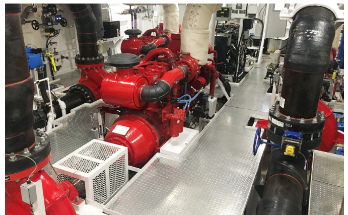
Logan LC-318's inside the St. Francis Engine Room and Pumping Station
